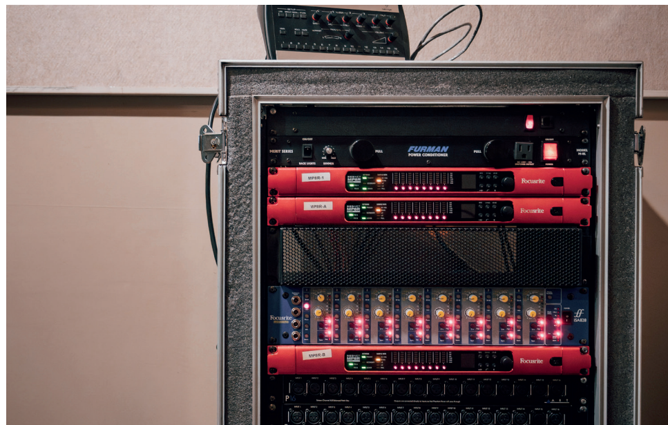
Gear rack in use at the five-studio production facility at the Department of Music Industry Studies at Loyola University New Orleans, featuring Focusrite RedNet MP8R eight-channel mic pre and A/D converters
